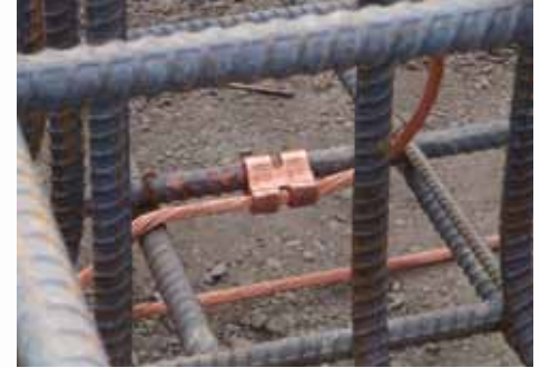
Grounding wire to rebar
