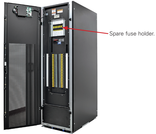
Figure 12. RPP with QSCP chassis and spare CUBEFuses in holder. Courtesy Liebert® FDC™ power distribution cabinet from Emerson Network Power™.
