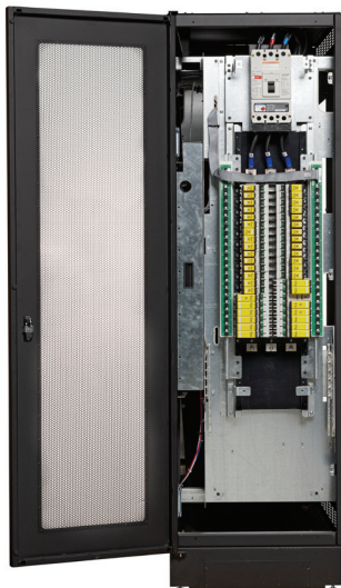
Figure 10. Eaton RPP with QSCP chassis.
