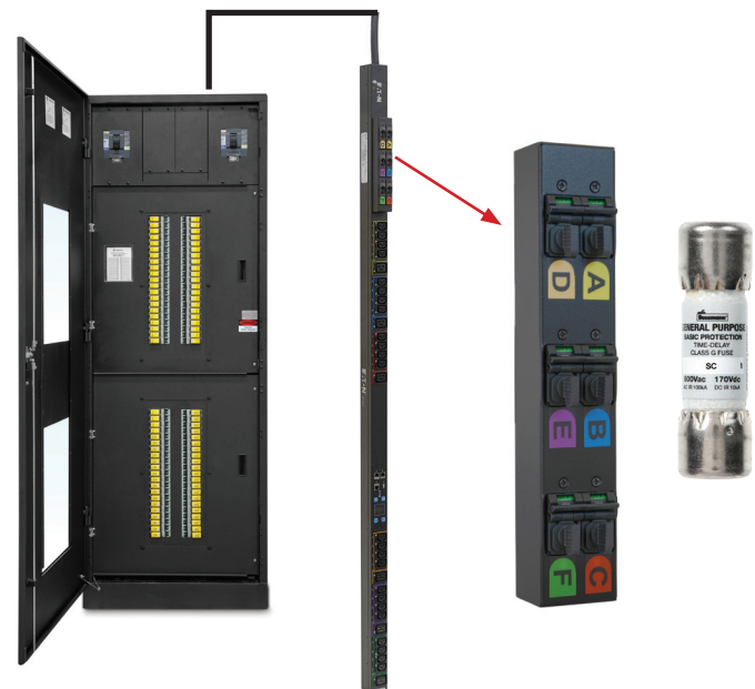
Figure 8. RPP utilizing QSCP with CUBEFuse feeding Eaton ePDUs utilizing CCPLs with SC fuses.
